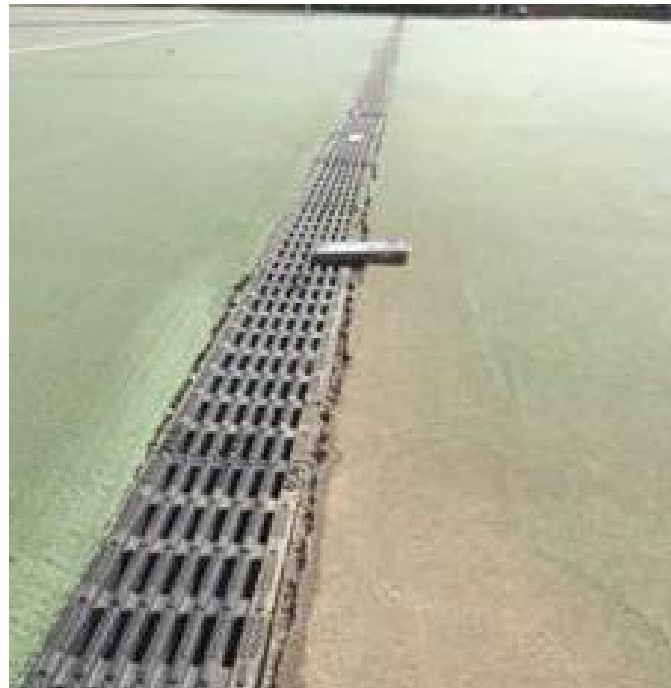
Figure 5 Courts linear drainage grate, engineering report advises that inadequate court drainage has aided to surface failure.
