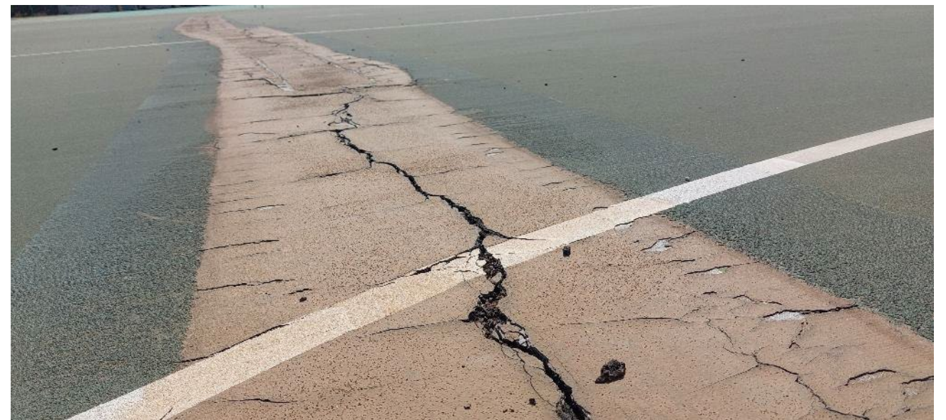
Figure 8 Evidence of surface cracking through repair work.
