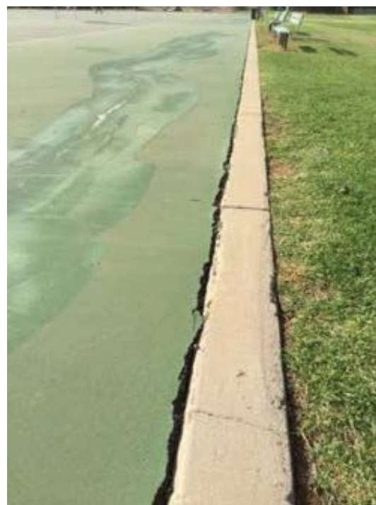
Figure 6 Courts concrete edging illustrating separation and subsidence from court surface.
