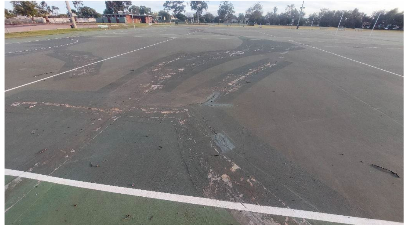
Figure 7 Existing court condition showing previous repair work.
